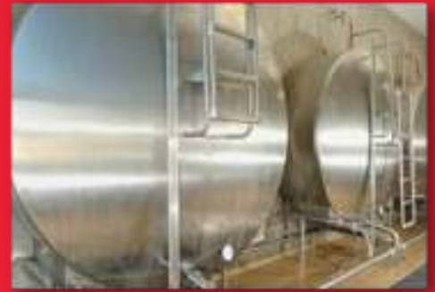
Pressure vessels & Storage vessels
